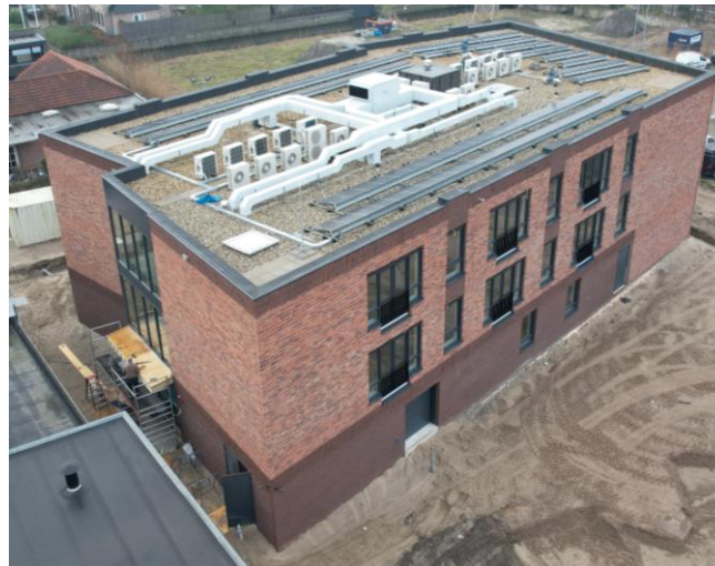
Figure 23. Aerial view of Droom je Thuis Foundation, including rooftop technical installations and PV system
