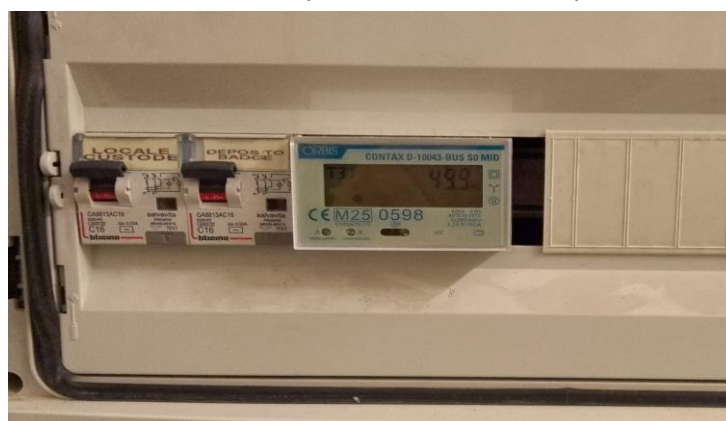
Figure 45. Installed electricity sub-meter for energy consumption monitoring
