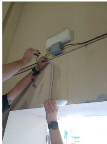
Figure 16. Counting people sensor installation
