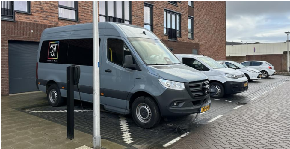
Figure 24. Zaptec Pro charging station for the Mercedes eSprinter at Droom je Thuis Foundation
