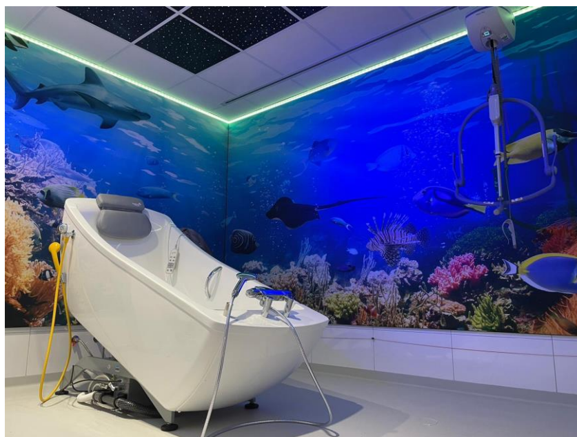
Figure 14. Detail on ceiling lifts installed in a bathroom
