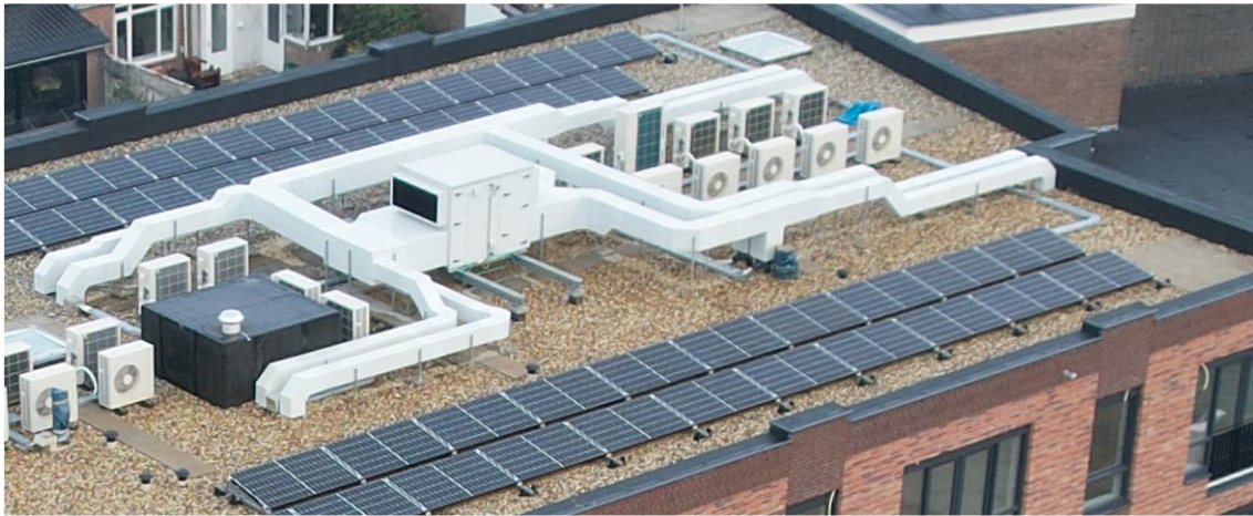
Figure 13. Technical asset on the roof of the building
